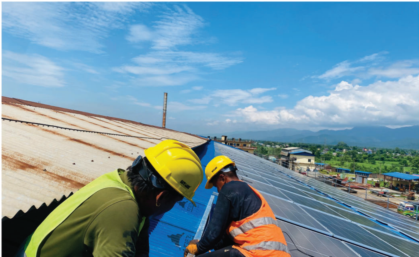
Technicians install solar panels at Laxmi Steels Industry as part of the GRIPS2 project — a catalytic lighthouse initiative showcasing how smart solar and storage systems can revolutionise Nepal's industrial energy landscape.
